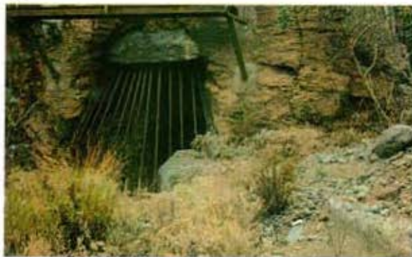
61. LAS PALMAS, CANARY ISLANDS. An arroyo is part-blocked by concrete/stone barrier on right, and bled off via a coarse trash screen to tunnels ( galeria ) and cave storages linked to irrigation systems at lower levels.
